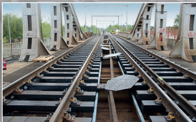
KLP® Hybrid Polymer Bridge Sleepers, Gent (Belgium).
